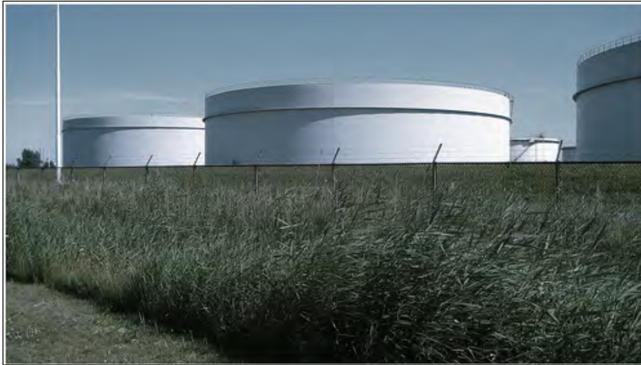
Figure 2-13: Typical Fuel Storage Facility
